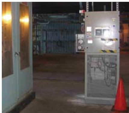
StableFlow hydrogen control system at FPL's Riviera Plant
